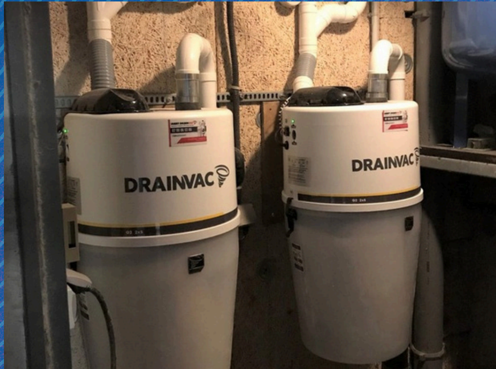
CENTRAL VACUUM SYSTEM
